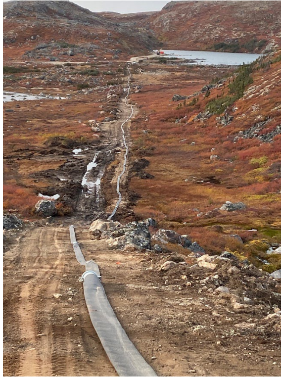
Photo 1: Kangiqsualujjuaq refill emergency pipeline laid out of constructed trail – source lake (Lake Ellsie) in the background with the pump visible on the shore.
