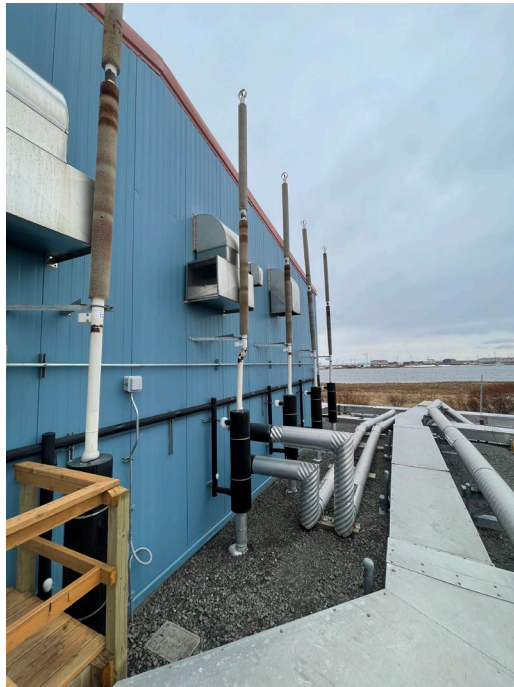
Figure 1. Hybridized sloping evaporator thermosyphon actively cooling the subgrade soils underneath the structure on the west side of the building in May of 2022.
