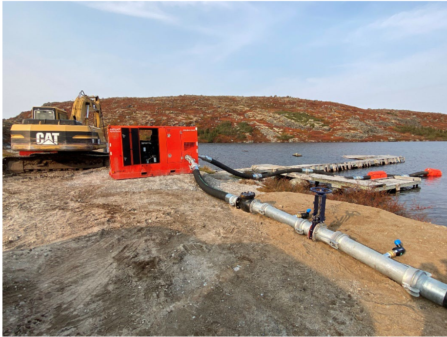
Photo 3: Pump and intake system in place on source lake (Lake Ellasie) with connection to the refill pipeline.
