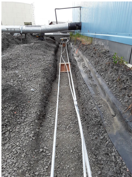
Figure 2. Attaching the ground temperature instrumentation to the flat-loop evaporator thermosyphon on the southern side of the structure in the summer of 2021.
